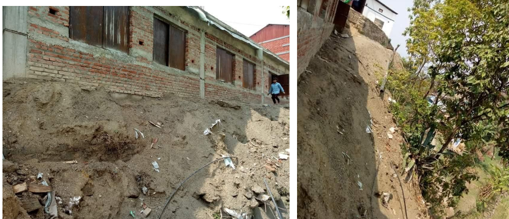
Figure 2: More pictures showing the need to provide levelling, retaining walls, and compound walls
