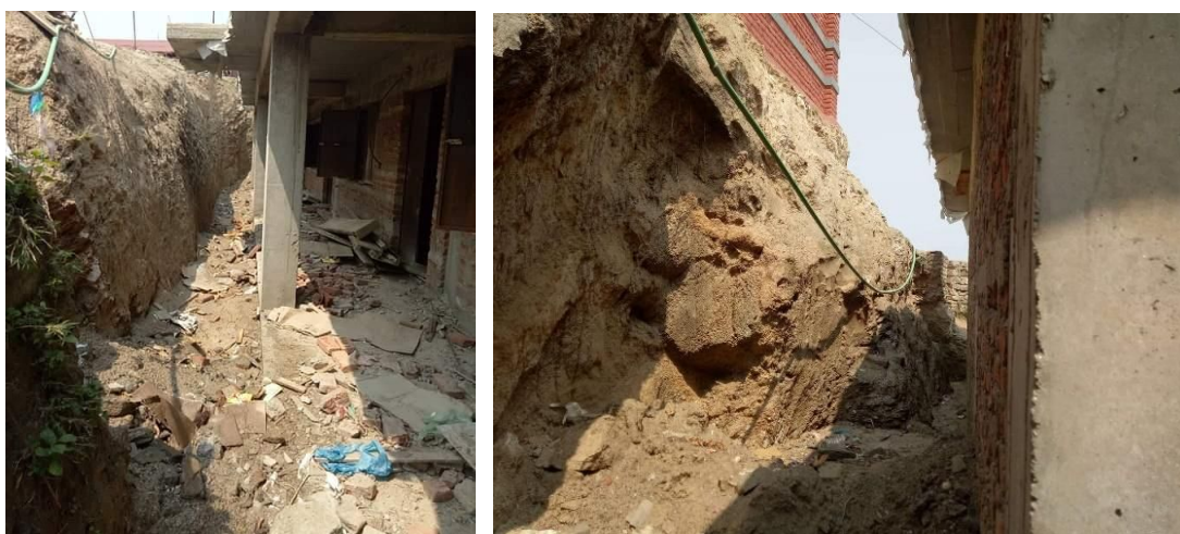
Figure 3: Immediate need for the retaining walls to be constructed in front and side of 6 roomed building
